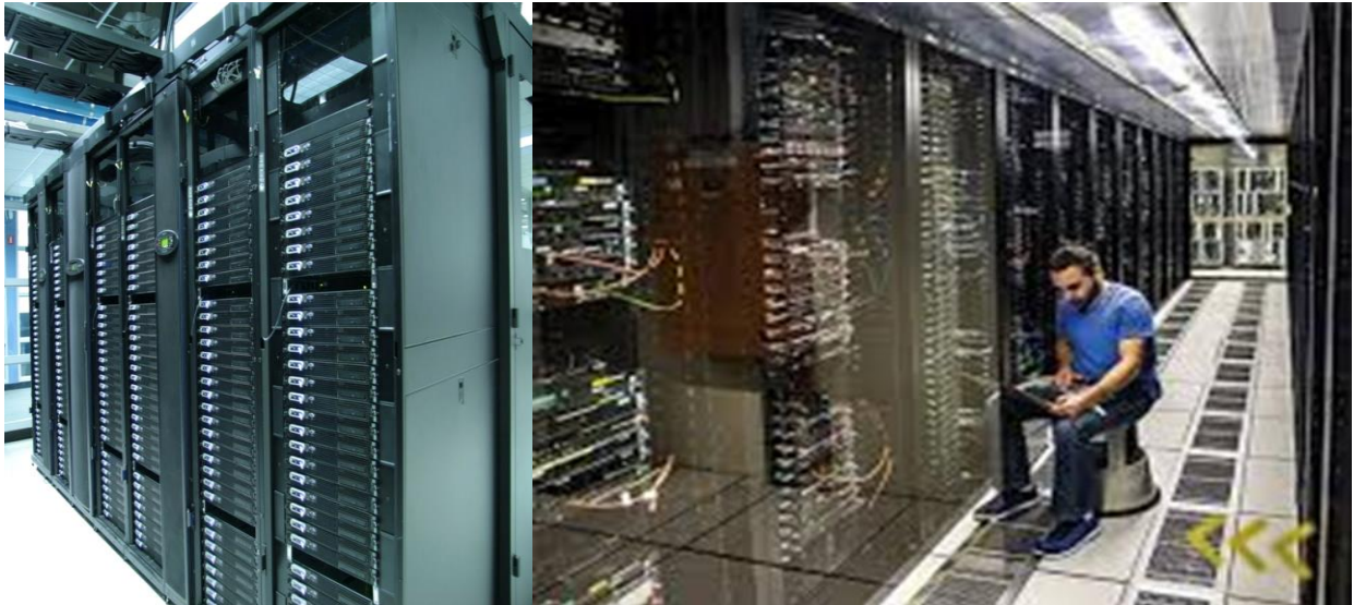
Fig.1.3. Data center example.
