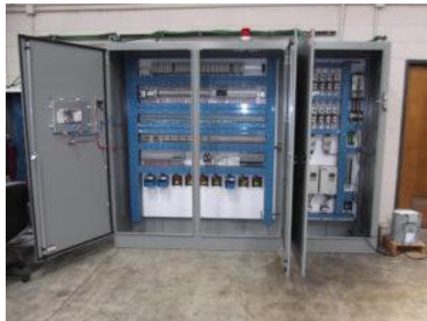
Figure 3.20 Electrical Control Panel – Internal
